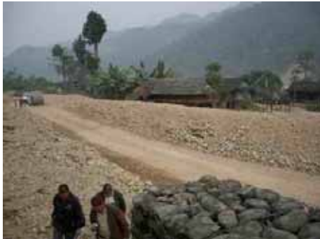
A scene after the removal of debris at Section I of the Sindhuli Road
