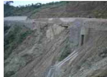
Damage at Section II of the Sindhuli Road
