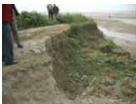
Damage at the Lakhandehi River
