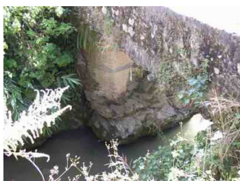
The substructure of the bridge is severely scoured.
