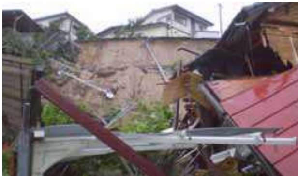
Slope failure hit a village. ( Ashiki, Chikushino City)
