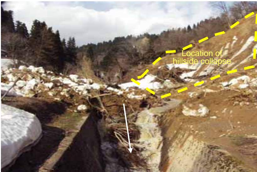
[April 23, 2005: hillside collapse] Place: Kizawa area, Kawaguchi Town, Niigata Prefecture Damage: A hillside collapse occurred in the area of 250 m wide and 70 m long. The channel of the Class A Matsuzawa River was clogged.
