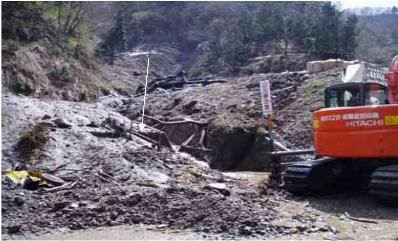
[April 23, 2005: hillside collapse] Place: Nigorizawa area, Nagaoka City, Niigata Prefecture Damage: A hillside collapse occurred in the area of 100 m wide and 300 m long. Sediment flowed out to the Kashiwazaki-Takahama-Horinouchi line of the prefectural road, closing to traffic temporarily.
